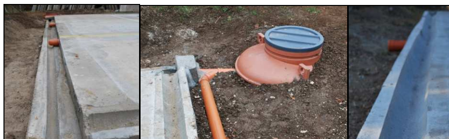
Fig.13 - Gutters and marginal leakage collection
