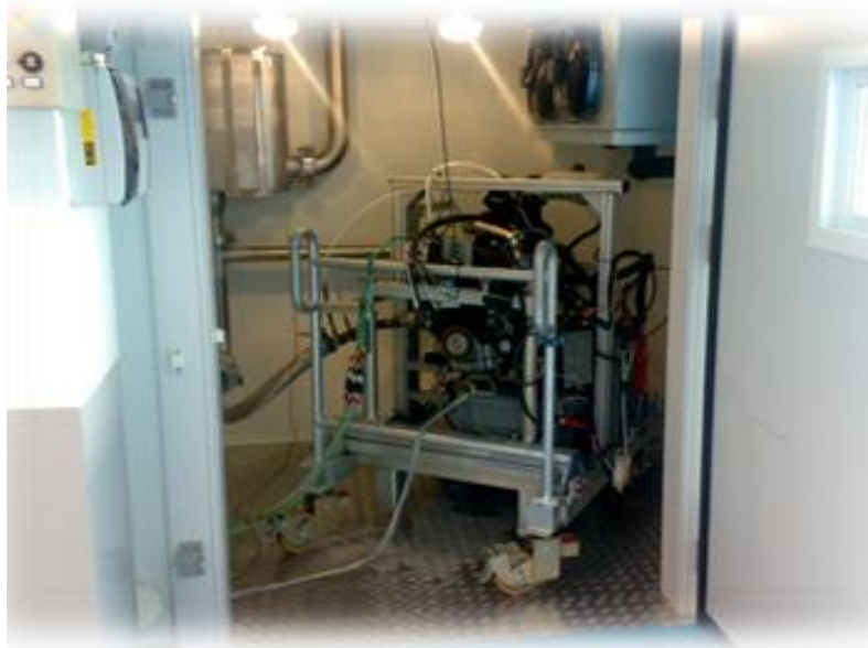
Fig. 1 – Cold Chamber / Camera Frigorifică
